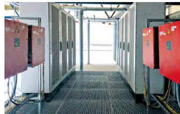
The energy storage system comprises switchgear cabinets, battery modules, inverters and plenty of cables.
