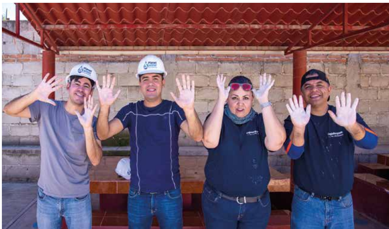
Employees from EagleBurgmann and the Planet Water Foundation installing an AquaTower in Quéretaro, Mexico.
