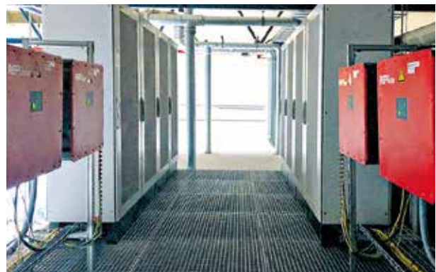
The energy storage system comprises switchgear cabinets, battery modules, inverters and plenty of cables.
